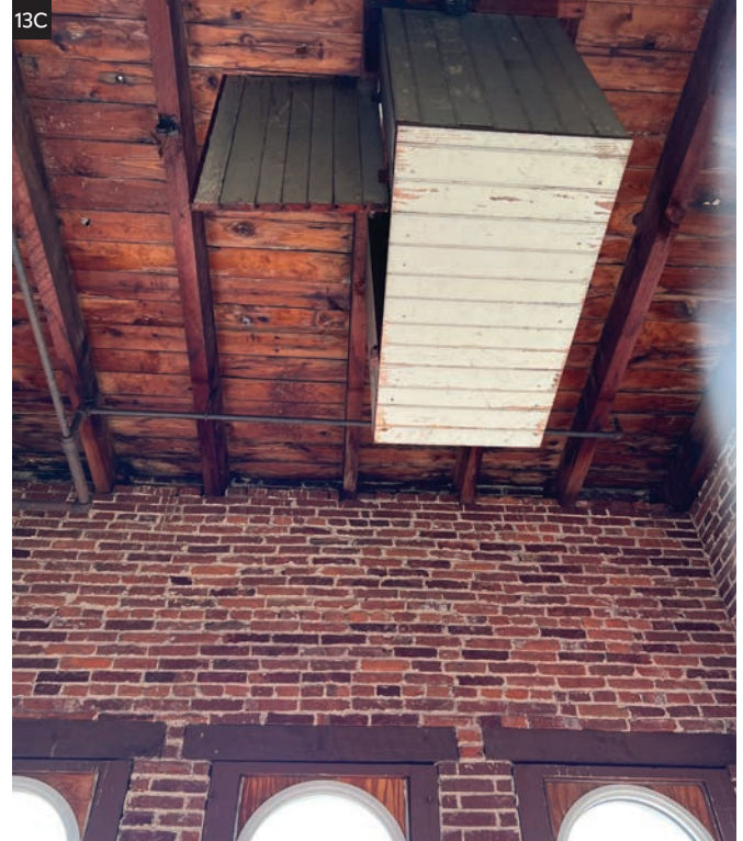
Figure 13C. In the East Tower, the wood case is still there, with the access door that protected and allowed the 8' pendulum to swing below the top floor of the tower room where the clockworks were mounted. There is no such case or provision for one in the West Tower. PHOTO BY MELONIE MURRAY.
