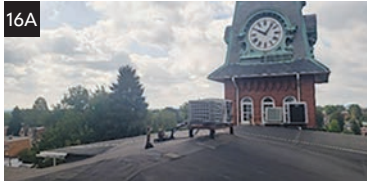
Figure 16A. Getting to the tower clocks at Hamilton is difficult and can even be dangerous, requiring you to first walk across a portion of the roof. B. You must then climb through a tower window onto steps into the tower's first level. C. To access the second level, it requires a person to climb a steep ladder to access the clockworks.
